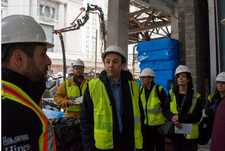
Council Member Powers tours the construction site of One Vanderbilt in East Midtown.
