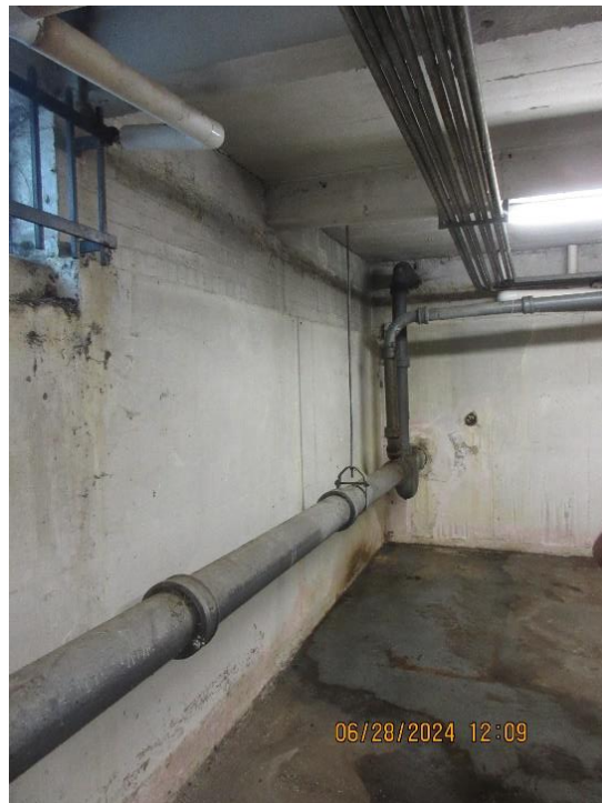
Photo 6 – Existing house trap located at Building NN
