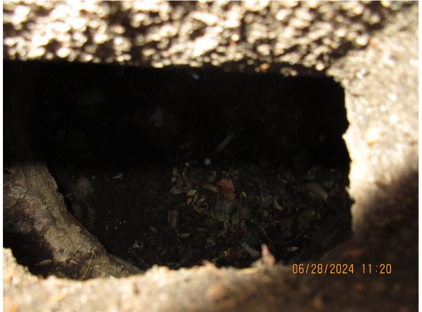
Photo 3 – Debris-filled catch basin in northwest courtyard
