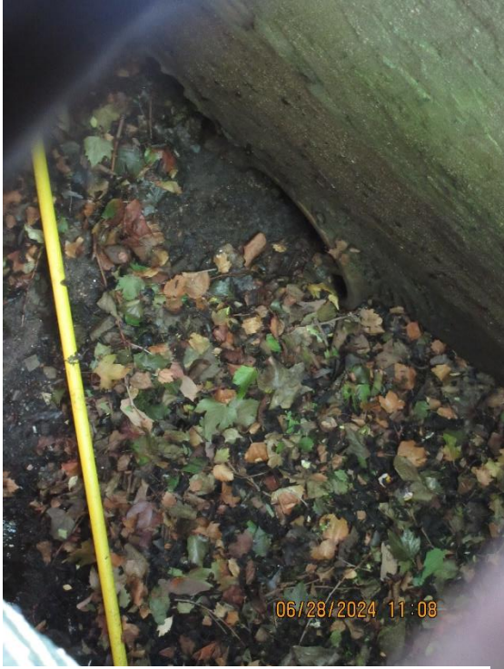
Photo 2 – Debris filled trench drain
