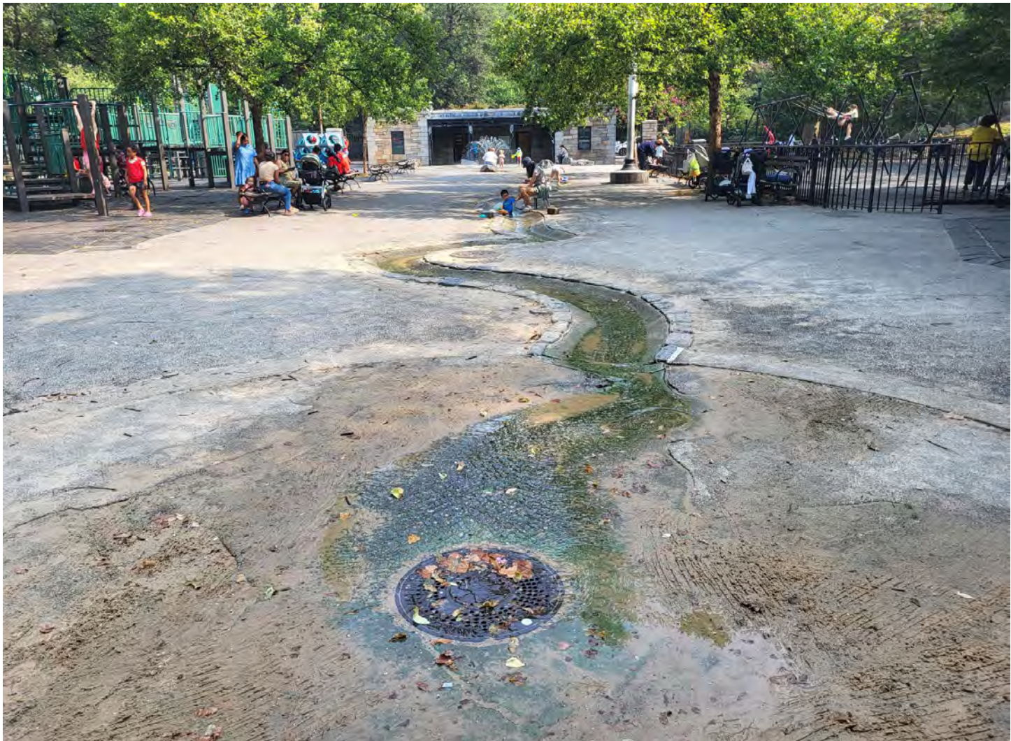
10 - Water runnel is in poor condition
